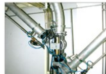
External Bypass Conveying Pipeline
